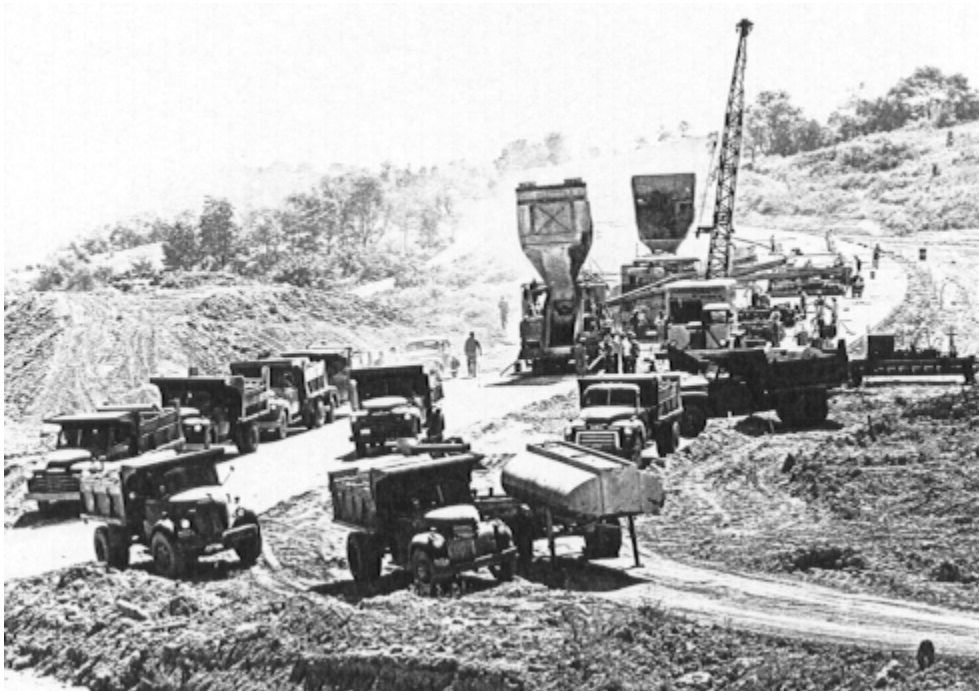
Penn-Lincoln Parkway under construction at the Campbells Run Road interchange in 1951. (Clyde Hare)
